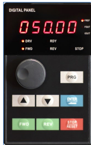
Figure B2 Control Panel
